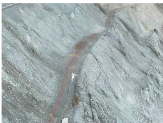
图6 下部单台阶微型桩方案现场治理照片 Fig.6 Site management photos of lower single step micro pile scheme
