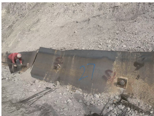
图5 上部边坡长锚索+钢板方案现场治理照片 Fig.5 Site treatment photos of upper slope long anchor cable+steel plate plan
